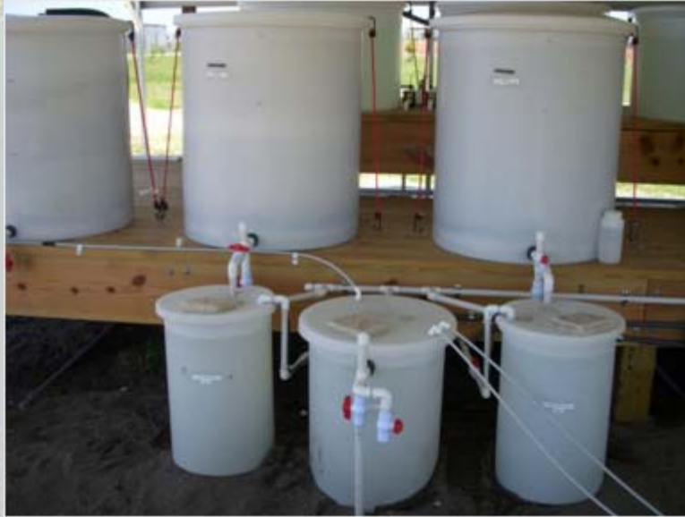
Stage 1 Recirculating Biofilters
