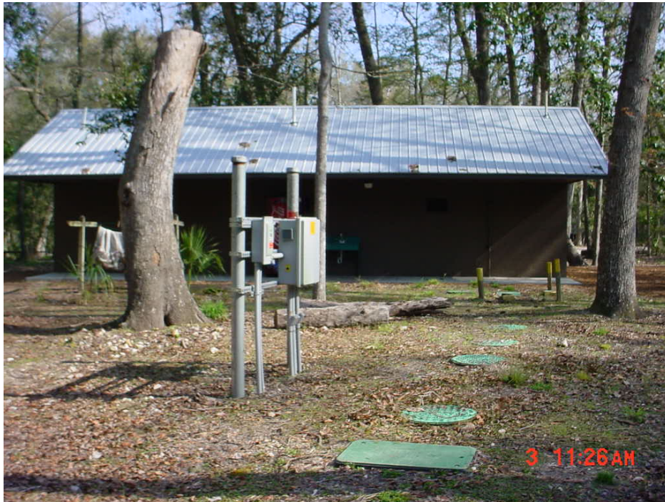
Picture 1. Hickory bathhouse on 03/03/2006. Dosing tank in front, septic tank to the left of posts.
