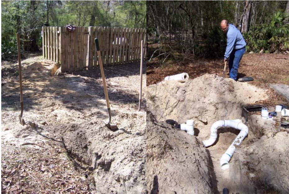
Picture 6. Magnolia II: Installing the return line from the ATU to the old drainfield, 02/24/2009.
