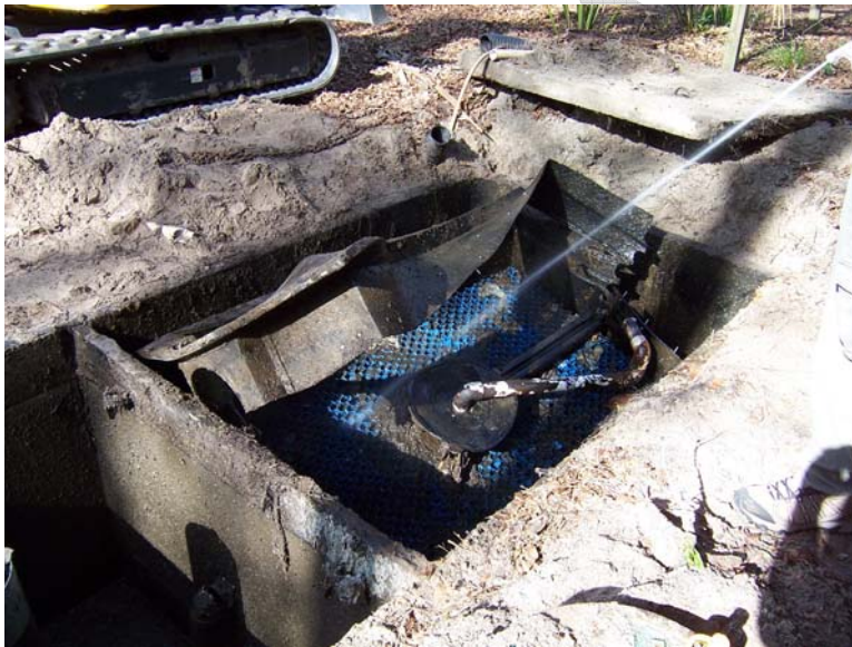
Picture 3. Broken treatment kit, due to increased weight from solids accumulation (note textiles) (March 2009)
