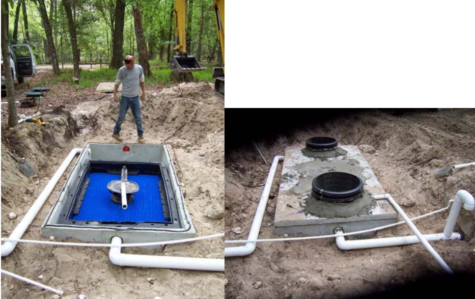
Picture 4. New treatment tank with treatment kit installed March 23, 2009
