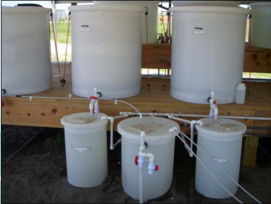
Stage 1 Recirculating Biofilters
