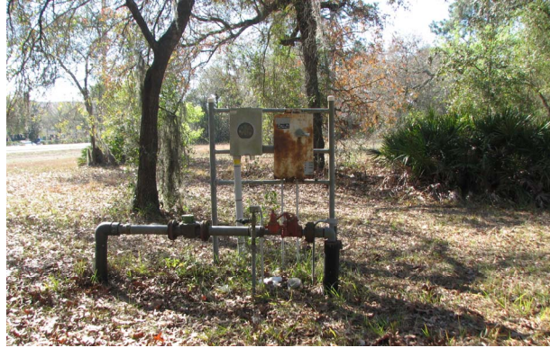
Figure 2. Water Well Pump and Controls
